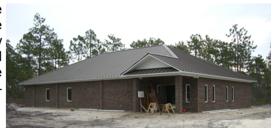
Exterior of New Hope Clinic under construction in Boiling Spring Lakes - March 1, 2010.
